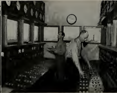
Leo Quayle and Harry Holmes, drydock control operators, at pump and valve controls which regulate amount of water in various compartments of the dock while ship is being raised or lowered. Dock has 16 compartments.
